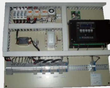
Main Relay Board
