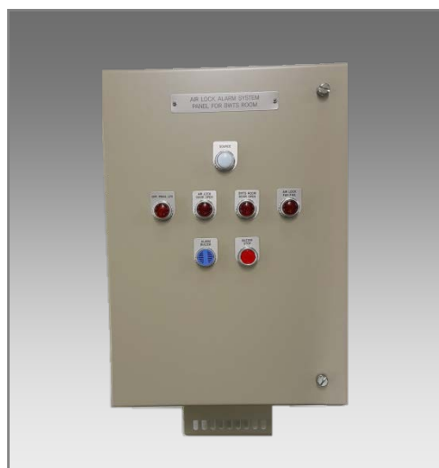
Air Lock Alarm Control Panel
